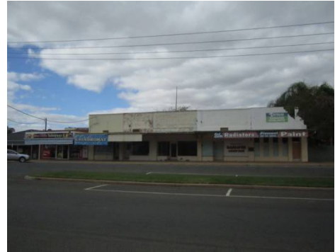
67-69 Ilex St. Sunshade panels to be constant height & fixed below original fascia
