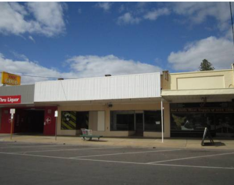
15 Ilex St. Remove upstand on awning edge as it obscures decorative parapets.
