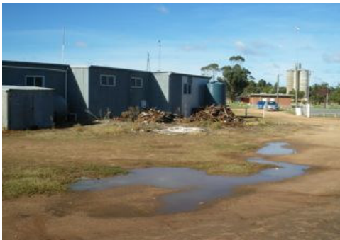
Rear of football / cricket change pavilion. Area in between pavilion and playground
